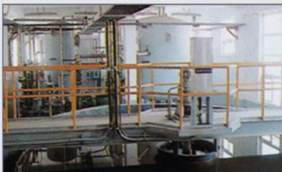
BIO REACTOR SYSTEM
